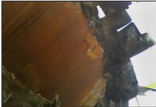
Transport pipe damaged by corrosive flue gas
